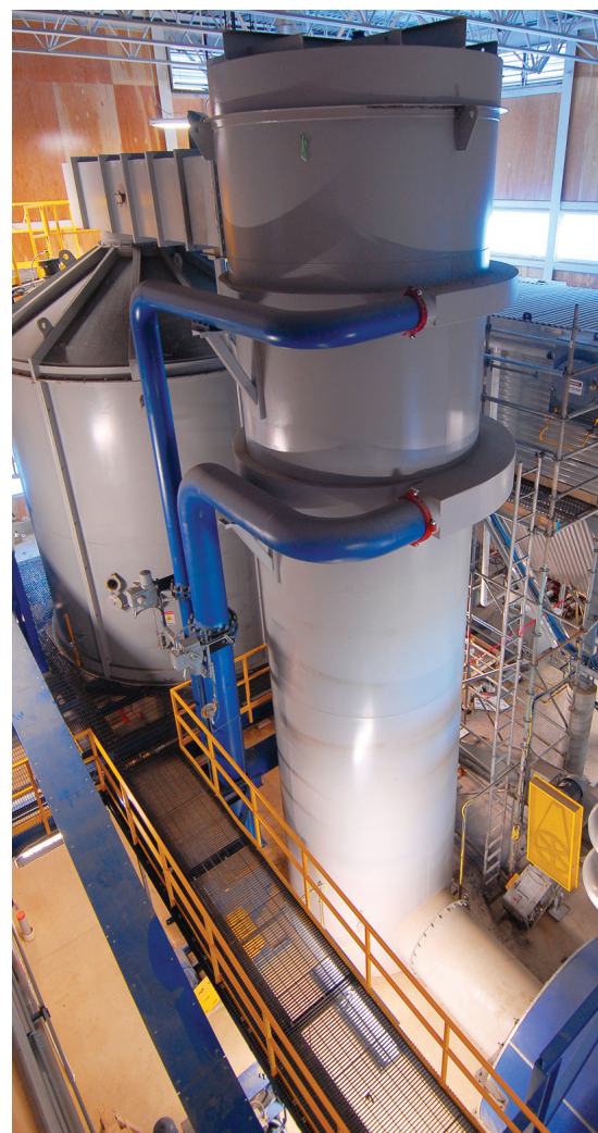
(1) Nexterra Systems's 5 MWt thermal gasification energy system at the University of Northern British Columbia in Prince George, B.C. (2) Nexterra's bioenergy project at The University of British Columbia will generate clean steam and electricity. (3) University of Northern British Columbia President George Iwama lights up the Nexterra gasification system that supplies heat for the Prince George campus.
