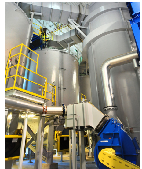
Nexterra's biomass gasification system at ORNL
